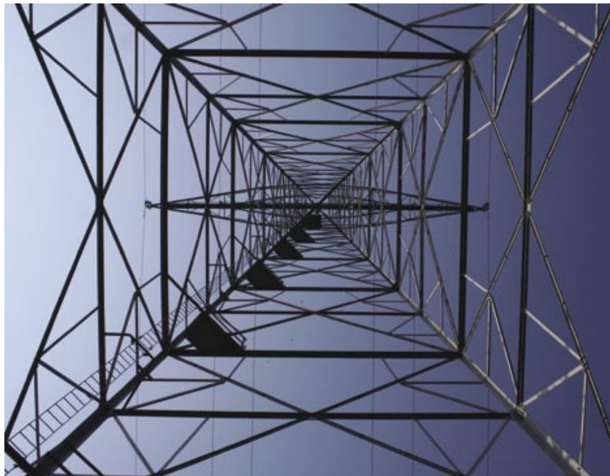
Power pylon on Marina
