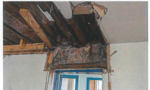
Door to T03 showing damage from partitions.
