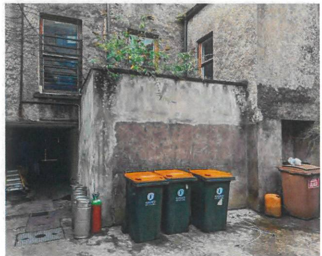
Rear yard showing passageway and one and two storey additions (middle and right).
