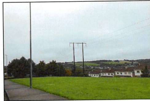
Plate 2- 10 Kilbarrý-Knockraha No. 2 110 kV Line crossing amenity grassland (GA2) within a residential area
