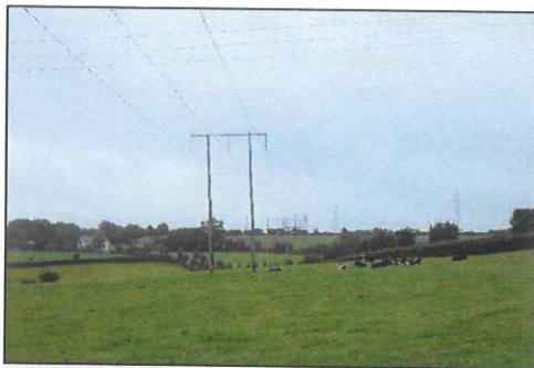
Plate 2-5 Kilbarry-Knockraha No. 2 110 kV Line crossing agricultural grassland (GAI)
