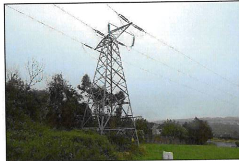
Plate 2- 12 Kilbarrý-Knockraha No. 2 110 kV Line within scrub (WS1) and amenity grassland within a residential area
