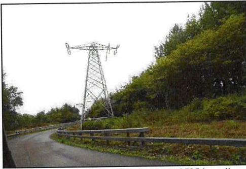
Plate 2- 9 Kilbarrý-Knockraha No. 2 110 kV Line adjacent to the roadway classified as Buildings and Artificial surfaces (BL3)
