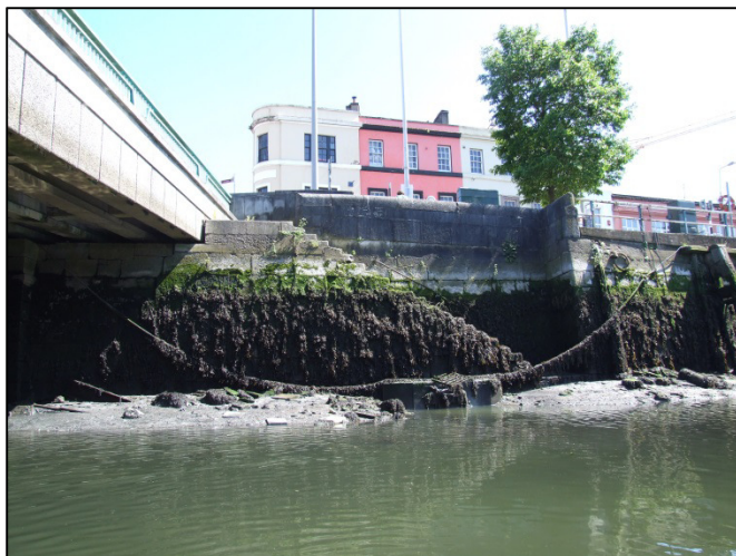
Plate 34: South-facing view showing masonry steps built as part of the original Parnell Bridge.
