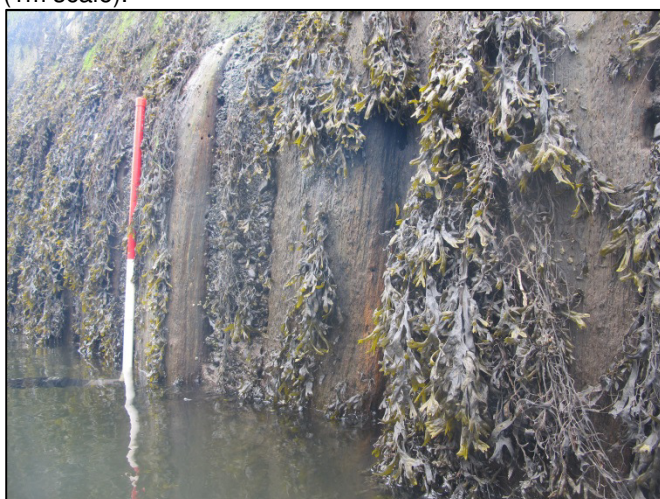
Plate 12: Example shot of timber piles set flush to the quay wall along Father Matthew Quay (1m scale).
