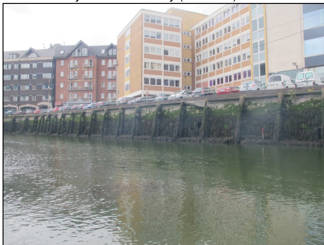
Plate 14: Northwest-facing view along eastern half of Morrison's Quay; taken at Low Water (1m scale).
