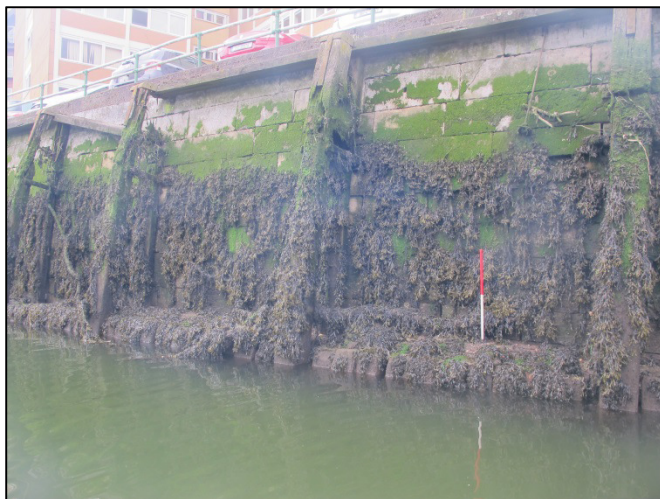
Plate 10: Northwest-facing view Morrison's Quay showing timber piles (Type 1) and concrete used to underpin sections of Father Matthew Quay/Morrison's Quay (1m scale).
