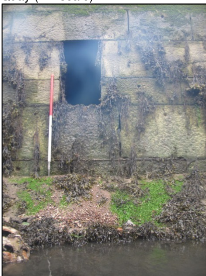
Plate 21: Example shot showing one of the larger rectangular drain features located along Father Matthew Quay/Morrison's Quay (1m scale).
