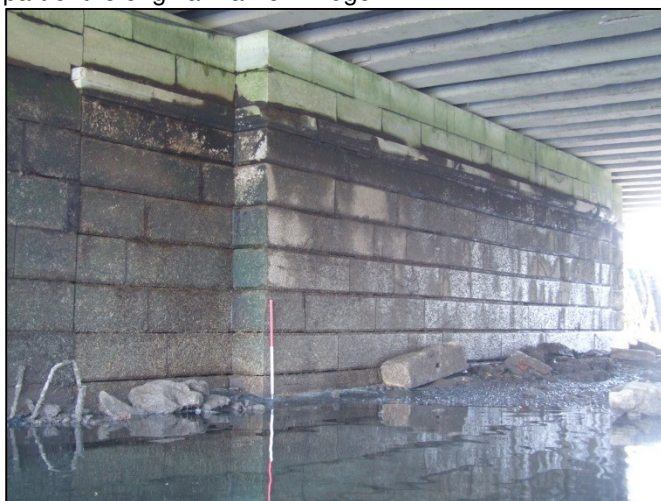
Plate 35: Northeast-facing view showing masonry forming a bridge abutment on the north side of the channel, located beneath the original Parnell Bridge (1m scale).
