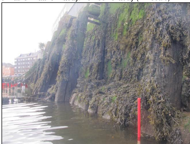
Plate 11: Example shot of timber piles (Type 1) used to underpin section of Father Matthew Quay/Morrison's Quay (1m scale).
