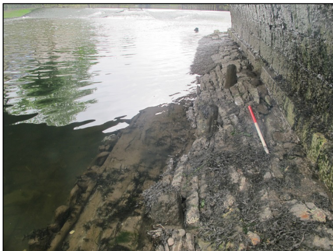
Plate 28: West-facing view timber shuttering and bridge foundations located on north side of archway at Parliament Bridge (1m scale).
