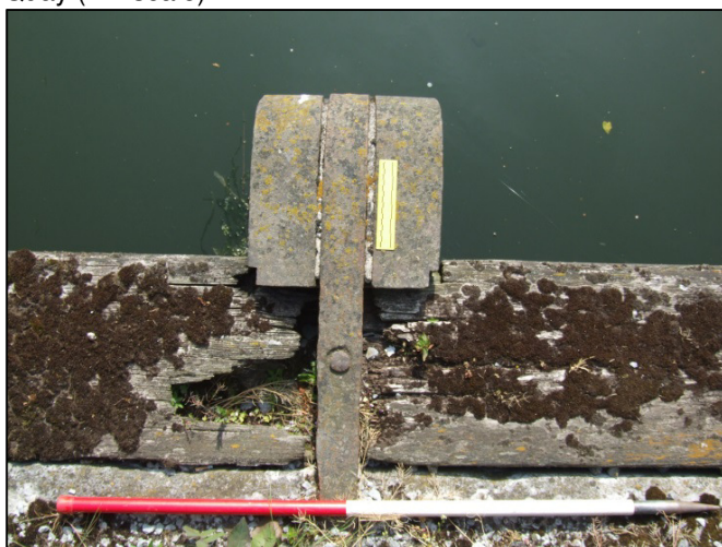
Plate 17: Example shot showing top-view of timber fenders used along Father Matthew Quay/Morrison's Quay (1m scale).
