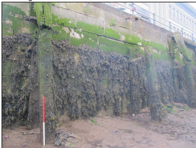
Plate 8: Northeast-facing view showing the fabric of the quay structure forming Father Matthew Quay and Morrison's Quay (1m scale).
