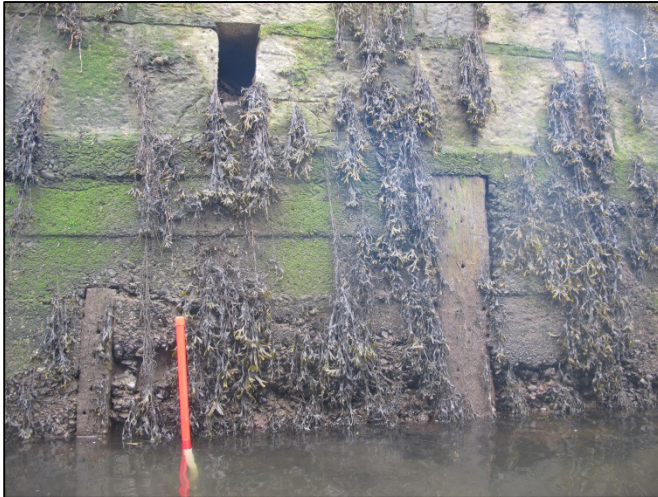
Plate 20: Example shot showing one of the smaller rectangular drain features located along Father Matthew Quay/Morrison's Quay (1m scale).
